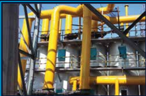
▲ Total Ducting of Gas Cleaning Plant
