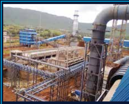
▲ 1.2 MTPA Pallet Plant Total Internal Piping & Ducting
