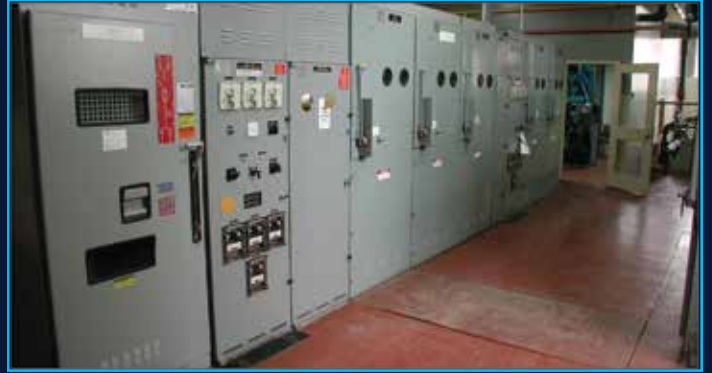
▲ MV electrical distribution room for SMS
