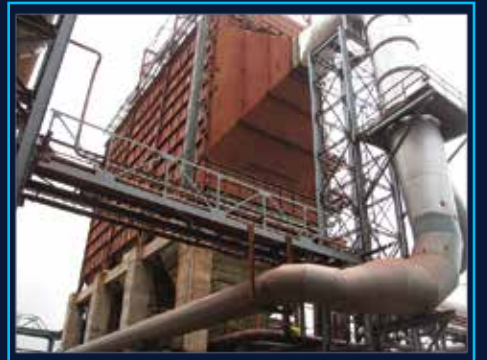
▲ Pollution Control System for Sinter Plant Material Handling
